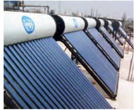
Solar water heating system in tanneries in Bangladesh
