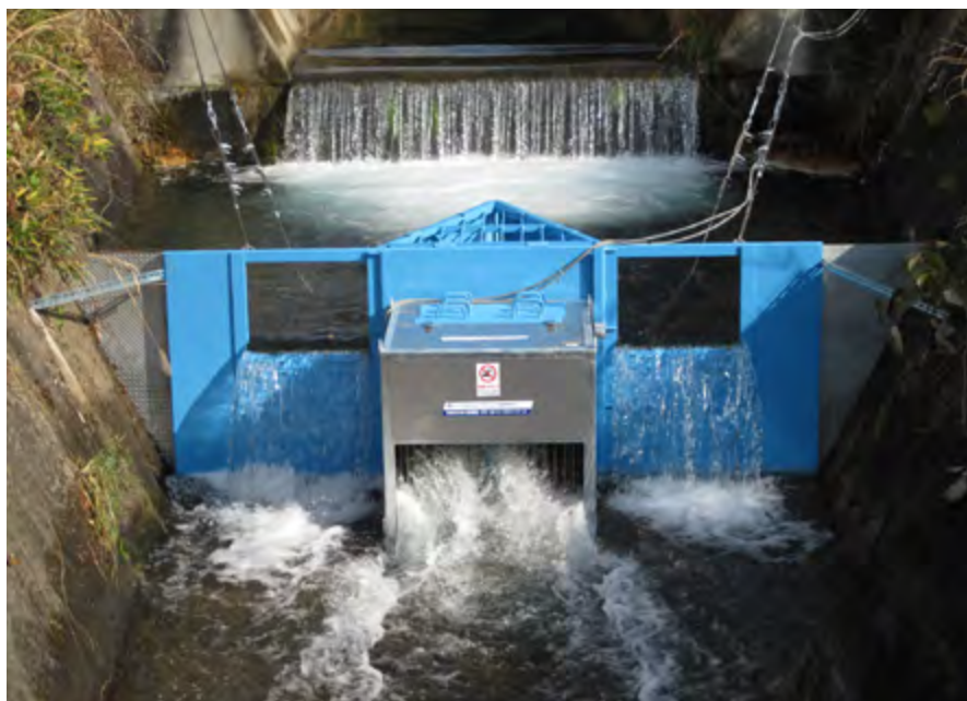
Ultra-low head micro hydropower installation in Mwea, Kenya
