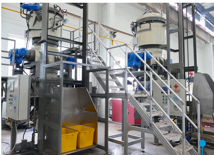
Installed autoclave equipment
